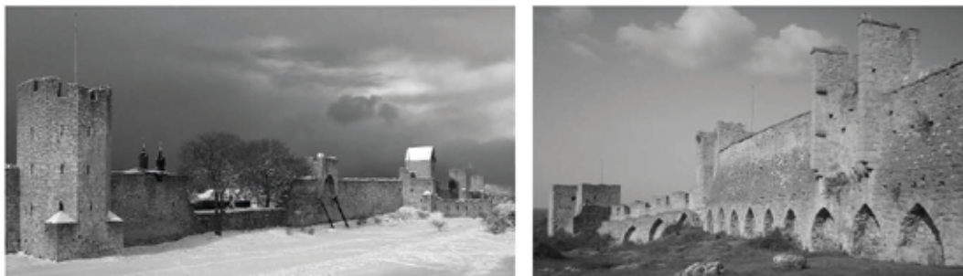
Figure 1. Visby City Wall seen from outside and inside. The smaller wall towers are riding on top of the wall. In many places one can see old collapses as well as different kinds of reinforcing structures.
