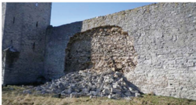
Figure 8. Visby City Wall in 26th of February 2012, a couple of days after the collapse.
