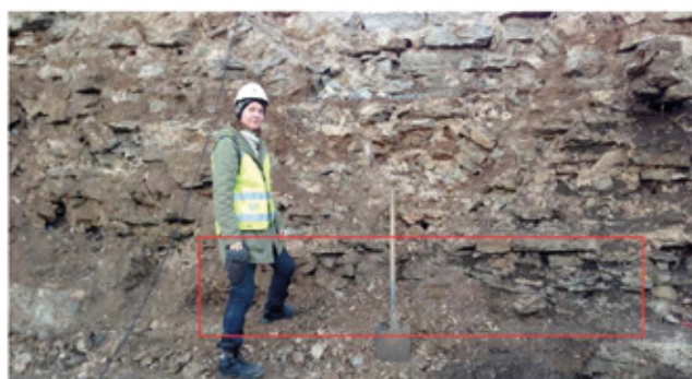
Figure 9. The area where the collapse probably started is a part of the wall where the masonry leaf was no thicker than a foot length, see the marked area. No binding stones were used in this part.
