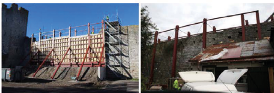
Figure 8: The temporary supporting steel structure, viewed from the outside during dismantling of the wall (left), and from the inside during erection (right).
