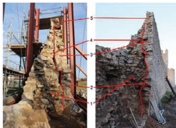
Figure 3: Two photos showing the same part of the wall at two different stages of dismantling of the collapsed part. 1) Lower core with clay mortar and no bond. 2) Thin outer masonry leaf. 3) Former parapet, now outer leaf of the middle part of the wall. 4) Upper core inside the parapet wall. 5) Top with solid masonry.
