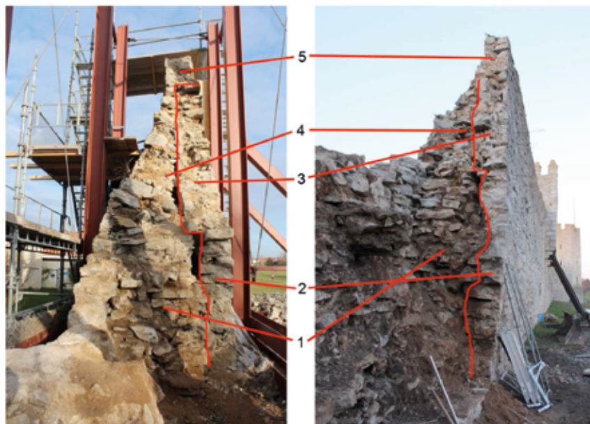
Figure 3. Two photos showing the same part of the wall at two different stages during dismantling of the collapsed part. 1) Lower core with clay mortar and no bond. 2) Thin outer masonry leaf. 3) Former parapet now outer leaf of middle part of the wall. 4) Upper core inside parapet wall. 5) Top with solid masonry.
