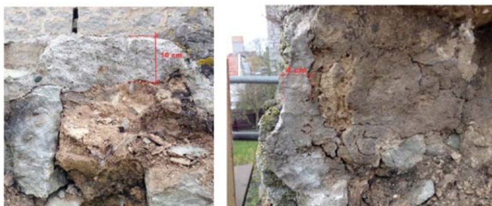
Figure 5. The first picture is showing the concrete cover on top of the wall, and directly beneath it is the type (c) mortar. Here this mortar was more deteriorated and more wet in approx. half a meter from the concrete layer than it was in general – not surprising for a 700 year old lime mortar situated on top of a wall. The second picture is showing the cement mortar covering the old lime mortar, showing the area of lime mortar just behind the cement as deteriorated in a thickness of approx. 5 cm.
