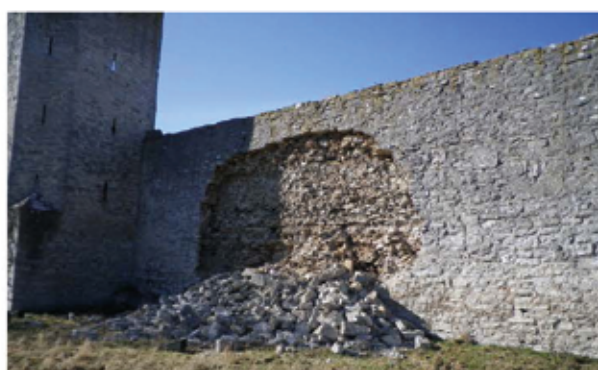
Figure 5: Visby City Wall in 26th of February 2012, a couple of days after the collapse.
