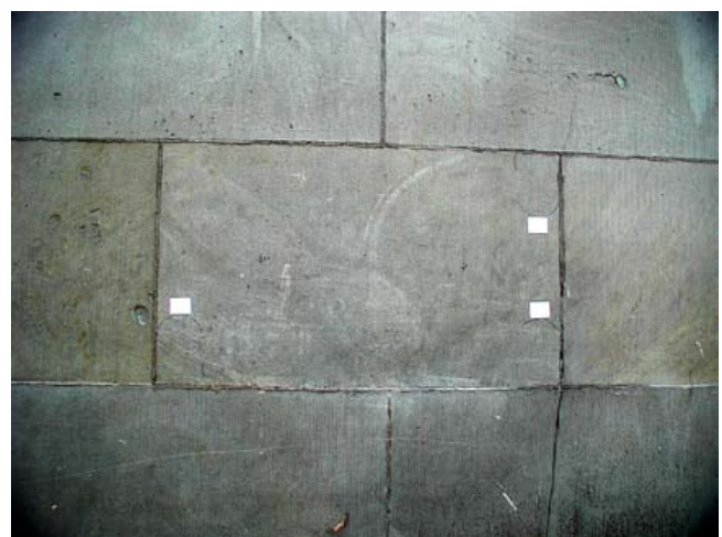
Figure 1. Labels attached for the granular disintegration test.
