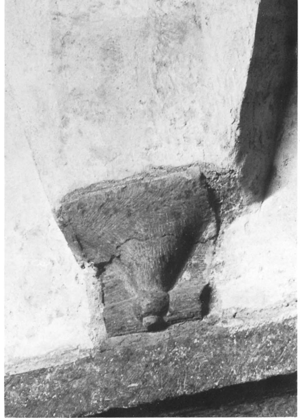
Vault brackets in the south (a) and north (b) in the south transept.
